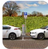
EV Charging Spots
